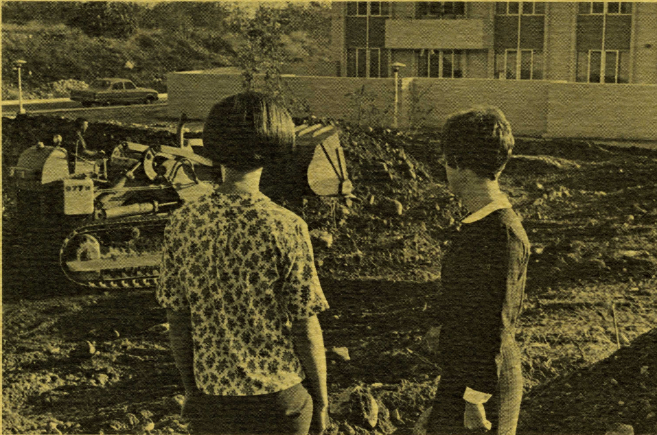
A big 'cat' churns the earth as ground is broken for Mead Hall and the dining center. Interested 'sidewalk superintendents' are students Elizabeth Shirley (left) and Judith Hanes.
